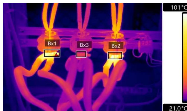
Fig.6. Thermogram of current transformer contacts
