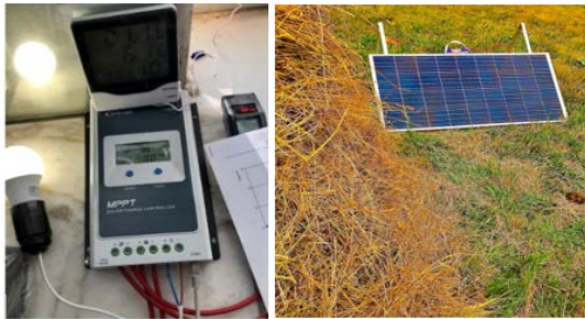
Fig. 7. The Components of solar power plant 150 W.
