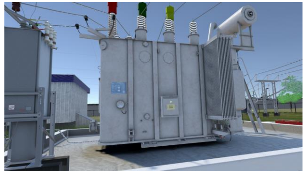
Fig. 1. Inspection of the transformer for defects.
