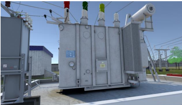
Fig. 3. Checking the operation of the algorithm for inspecting the box of a complete outdoor switchgear.
